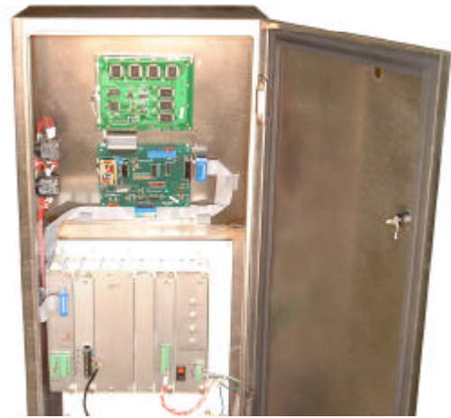
Internal View of Controller
