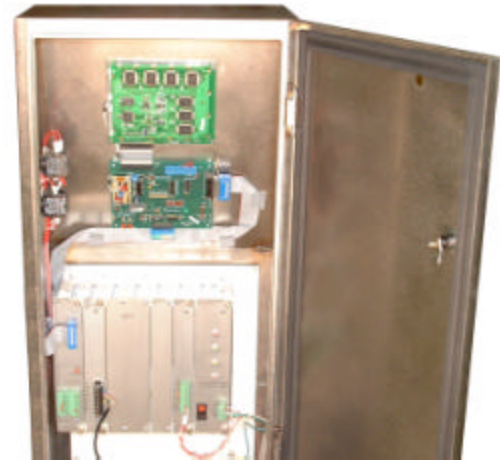
Internal View of Controller
