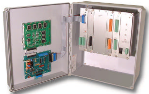
Internal View of Controller
